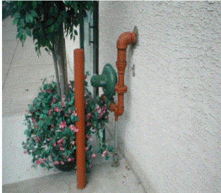
High Pressure Service Installed Outside Protected by Bollard & hidden By Planter
