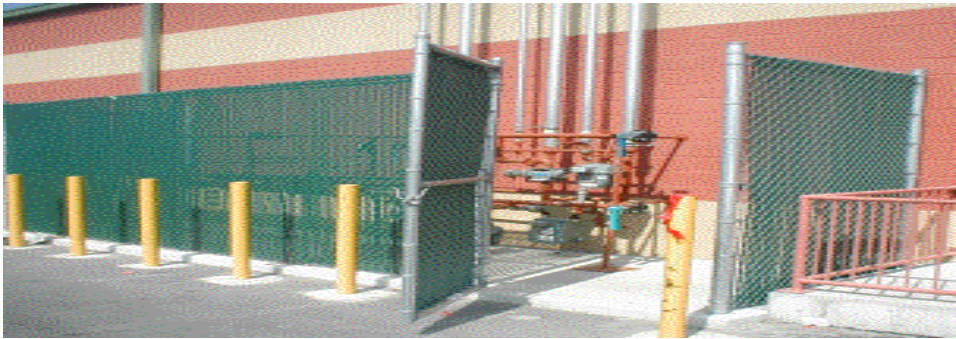
Light Commercial Multi-Metered Installation, Protected By Bollards and Fence In The rear of Shopping Center's Loading Dock.
